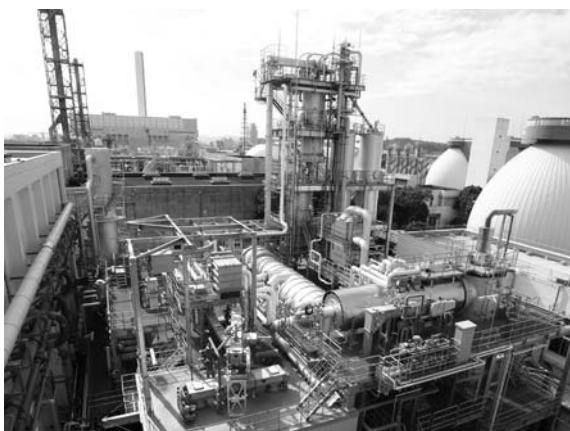
Photo 1 View of sludge to fuel conversion facilities
