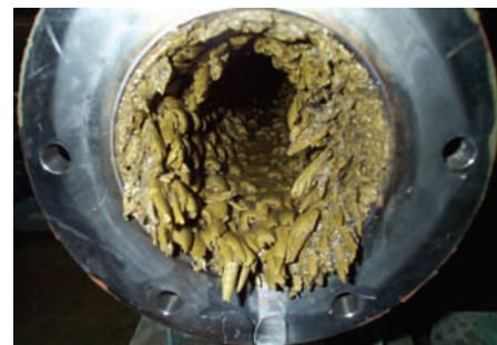
Fig.8: Gravity Concentrated Sludge Pipe Wall
